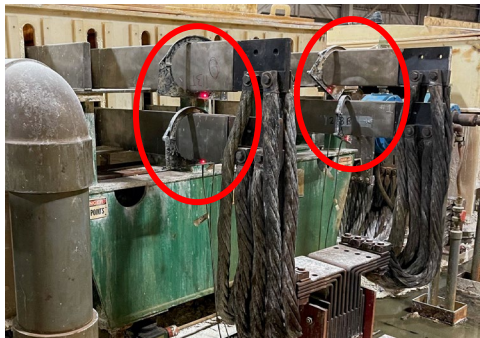
CPCO – Current Probe, Clamp-on Probe based on same technology and design with larger aperture, in use at an electrochemical plant.
